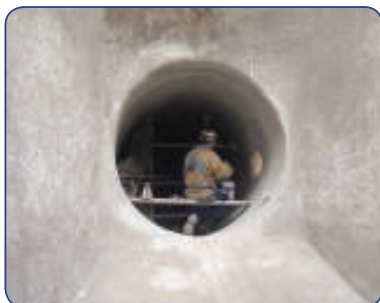
A Diamond Refractory worker performs a 100% demolition and refractory replacement on a waste heat cooler
