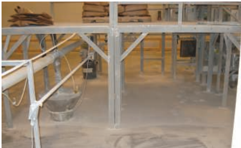
FIGURE 3. While housekeeping is important, facilities should focus on containing and collecting potentially flammable or explosive dust from the processes that handle or generate fine powdered materials. These include such common, seemingly innocuous materials, such as sugar, flour and sawdust
